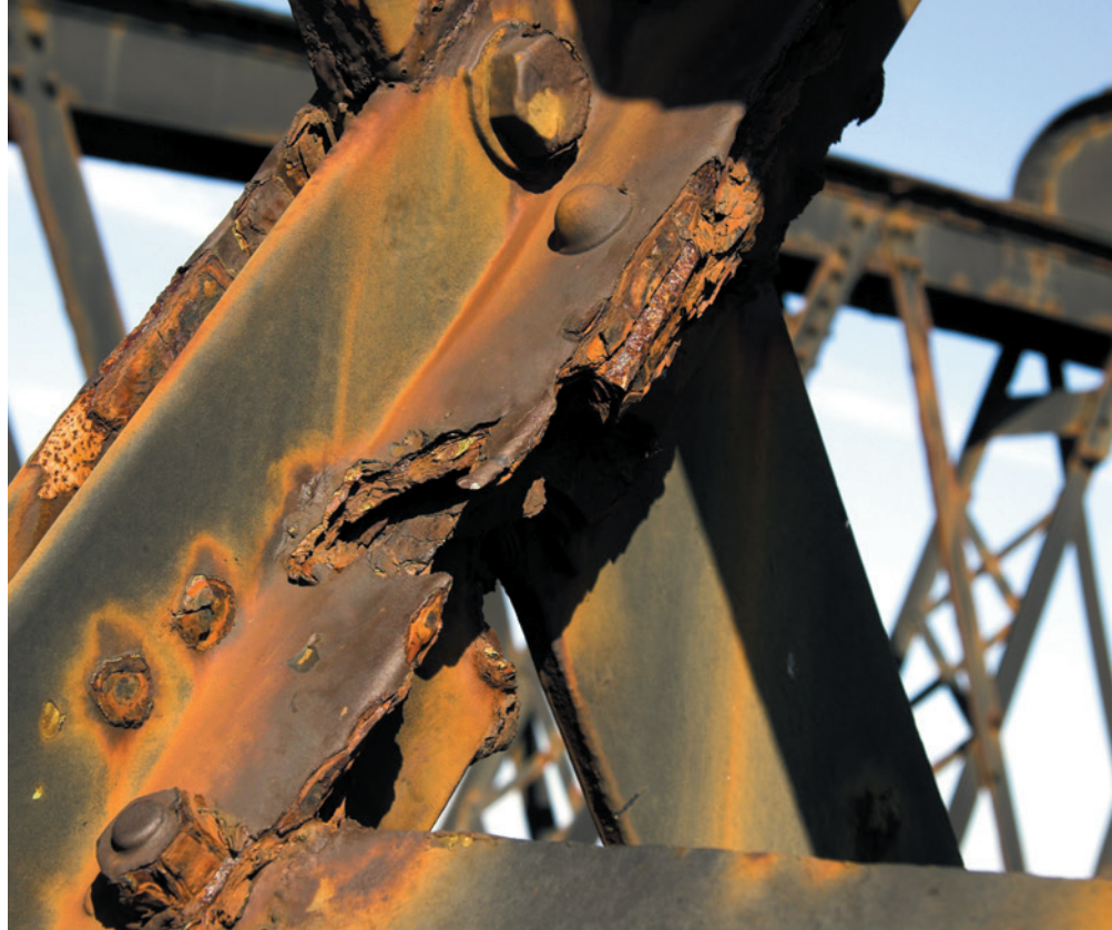
Corrosion costs around US$4 trillion a year globally.
